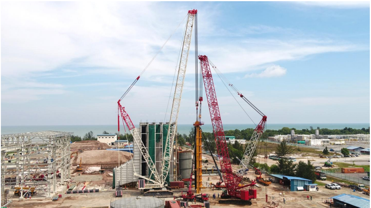
Executing tandem lifting, upending and installation of total 10 units 300 mt HRSG modules for the Tanjung Kidurong Combined Cycle Power Plant Phase 2 project at Bintulu by utilizing 650 mt Demag CC3800-1 and 550 mt Demag CC2600. The job involves non routine critical lifts under complex operations that require additional safety precaution, detail planning and under competent supervision.
