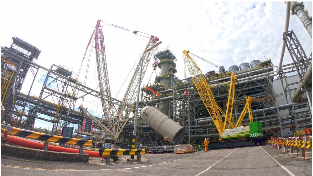
Transportation of Absorber Column from Bintulu Port to MRU Project Site using 10 + ½ PST/THP Goldhofer trailer and lifting utilising Demag CC3800-1
