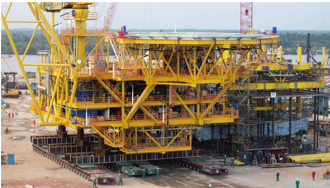
Shifting and Loadout of F28 DR-A TOPSIDE at Kencana HL Yard, Lumut; a project by Shell Berhad, on 21st-22nd June 2011. A total of 2 x 24 axes SLE and 2 x 12 axes ESE (72 axes Goldhofer trailers) were used to transport the topside weighing almost 2224 tonnes. The topside was shifted at a distance of 400 meters before crossing over to the barge the following day. 14 ballast pumps were used for ballasting.
