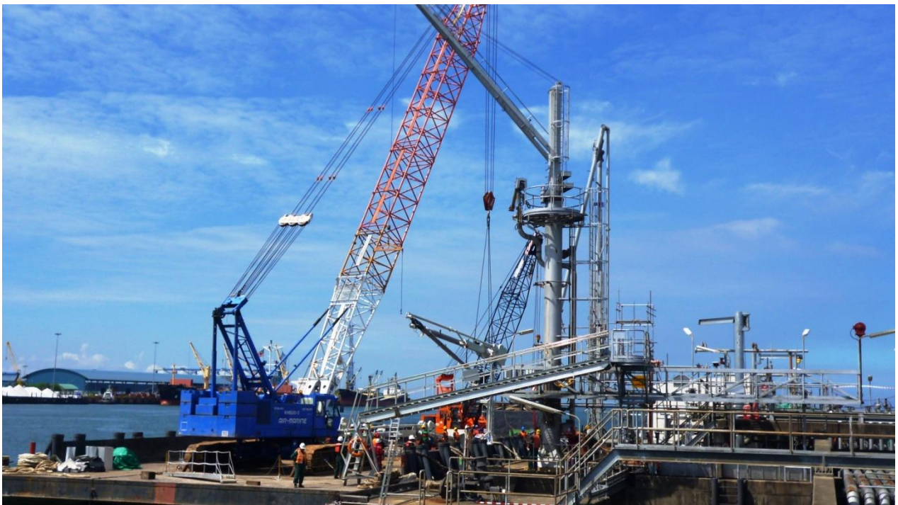
Erection of Sarawak SHELL Berhad's Loading Arm weighing 50 MT utilizing Hitachi KH500 as main crane and Kobelco 7450 as tailing crane.
