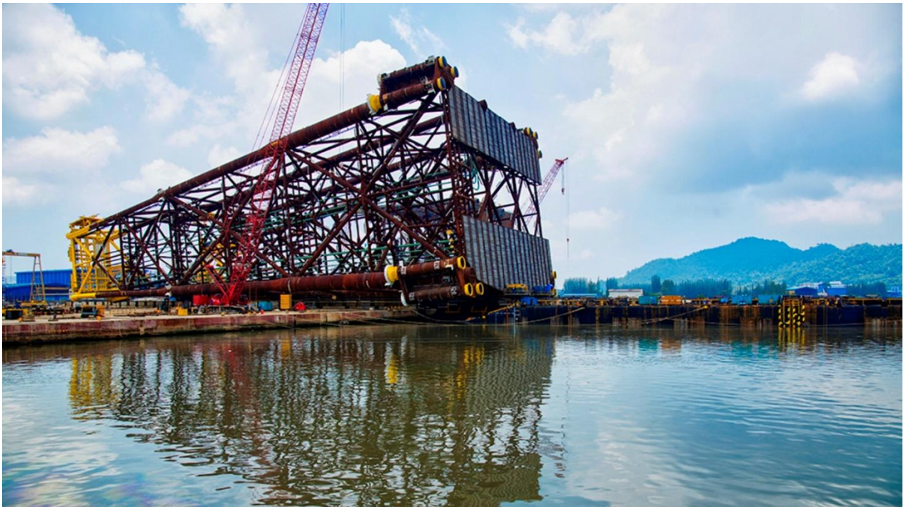
Loadout of Kebangsaan Petroleum Operating Company's KBB jacket weighing 14,400T utilizing 4 units of 735T capacity strand jacks to pull the jacket to transportation barge for our esteemed client, Sapura Kencana Petroleum Berhad.
