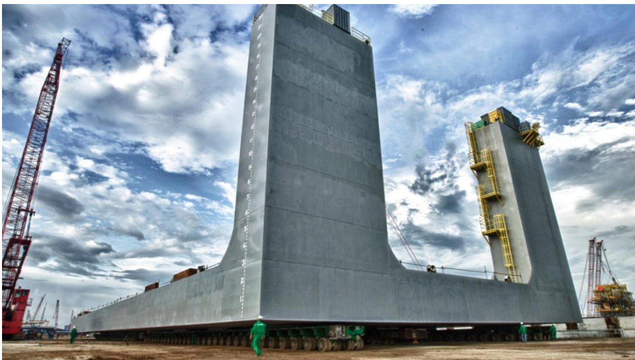
Shifting, Load Out and Barge Ballasting of Dockwise's Buoyancy Tank with combined weight of 4300MT utilizing 168 axle-lines Goldhofer Self-Propelled Modular Transporter at Kencana Petroleum's Yard, Lumut, Perak, Malaysia. After which, a separate operation of Load In, Shifting and Barge Ballasting is being carried out using the same equipments at Malaysian Marine & Heavy Engineering's Yard, Pasir Gudang, Johor, Malaysia
