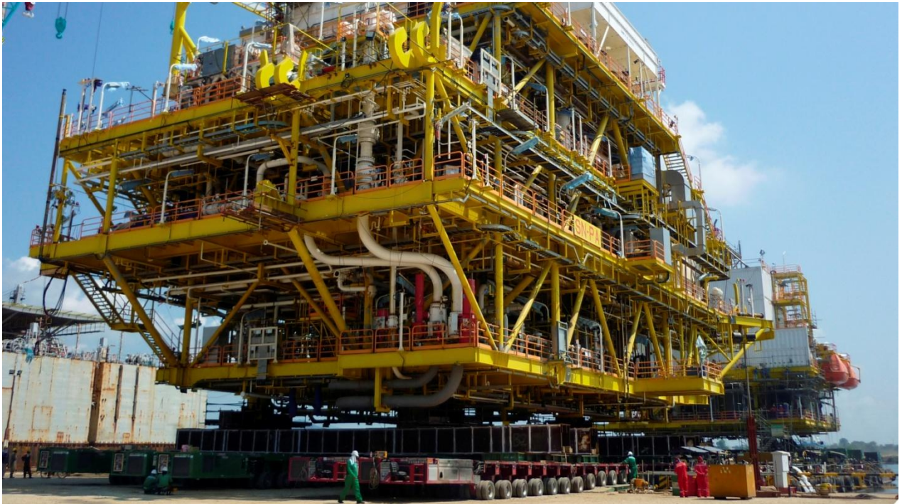
Shifting and loadout of SN-PA CPP Topside with combined weight of 3400MT from fabrication site onto barge in April 2013 for our esteemed client, Kencana HL Sdn Bhd at Lumut, Perak utilizing our Scheuerle & Goldhofer 120 axle-lines with 5 powerpacks.
