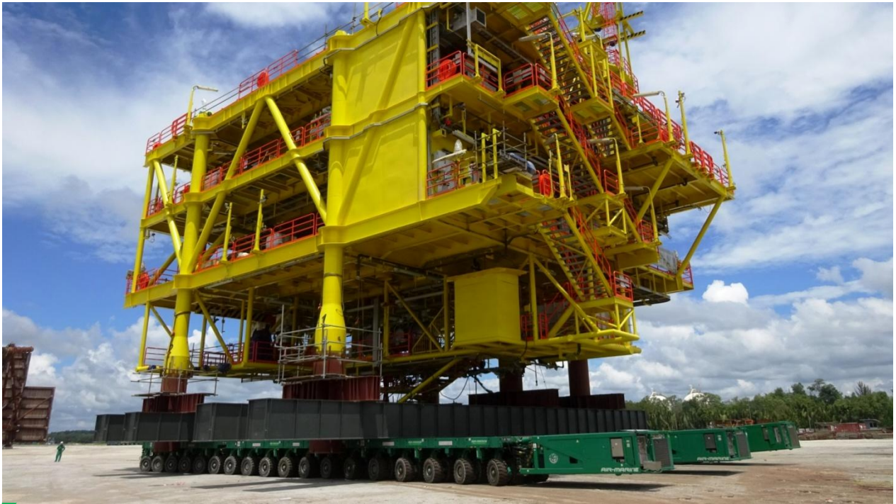
Shifting of 812Te BP-A (Bunga Pakma – A) Topside by utilising our 54 axlelines of Scheuerle 4th Gen. Self Propelled Modular Trailers (SPMT's) coupled with 3units hydraulic Powerpack units from the fabrication area to the quayside for our prestigious and distinguished clients Oceannight Sdn Bhd on the 11th of August 2017, at their fabrication yard in Kuching, Sarawak, for Repsol Oil & Gas Malaysia Ltd. The synchronised shifting operation lasted for around one hour and subsequently upon reaching the quay side, the Topside was loaded out to the already pre-ballasted 330' flat top ballastable barge by utilising 20nos of our diesel driven ballast pumps.
