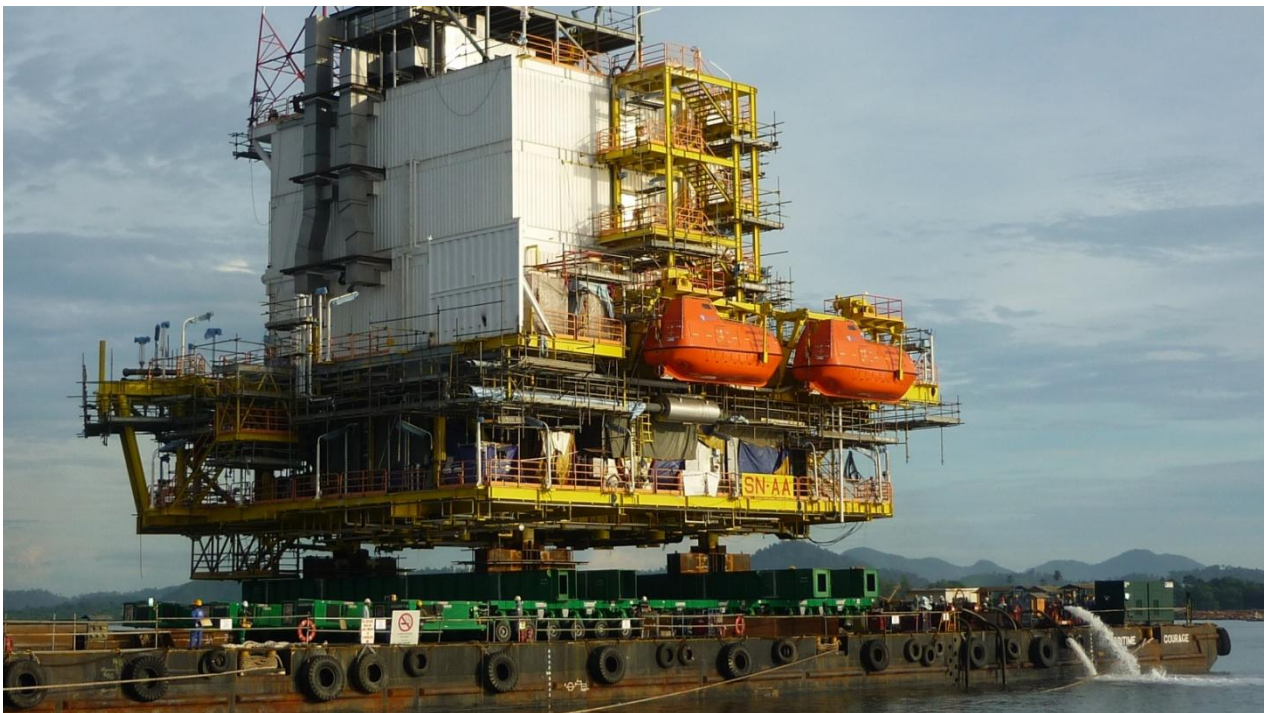
Shifting and loadout of SN-AA LQ Topside with combined weight of approximately 1900MT from fabrication site onto barge in April 2013 for our esteemed client, Kencana HL Sdn Bhd. For SN-AA LQ Topside's shifting and loadout, we utilized our Scheuerle's 72 axelines Self-Propelled Modular Transporter (SPMT) with 4 power packs. Combination of Scheuerle and Goldhofer's 120 axelines SPMT with 5 powerpacks is utilized for the shifting and loadout of SN-PA CPP Topside.
