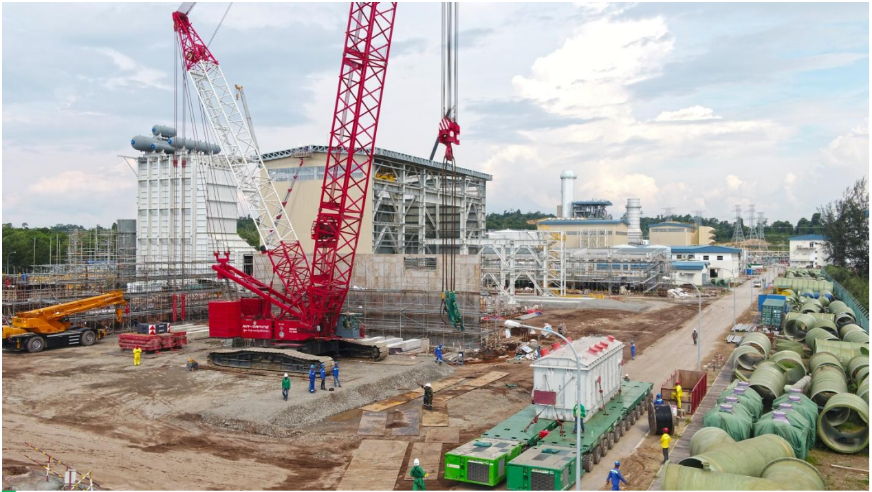
Transportation of transformer from Bintulu Port to TKCCPP Site using 24 axeline SCHEUERLE 4 th Generation SPMT and lifting of Transformer using Demag CC2600
