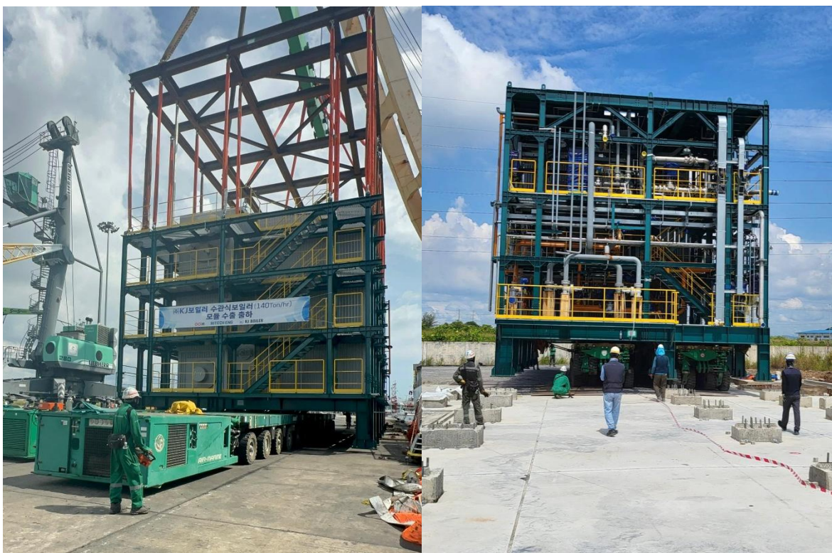
Direct receiving of 290T Boiler (20.5 x 9.96 x 10m) from Crane Vessel onto SCHEUERLE SPMT 12 x 2 (24) axline + 2 PPU. Transporting from Samalaju Port to OCI MP11 Samalaju Plant and final installation by jacking down onto Site Foundation.
