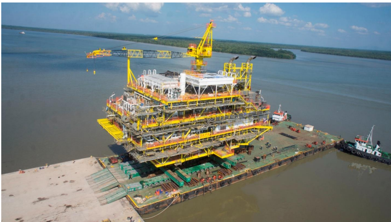
✓ The SA-PA Topside weighing 2408MT was fabricated at BDEWC yard in Kuching, Sarawak for Murphy Sarawak Oil Co. Ltd. AIR-MARINE utilised 96 axle lines of Self-Propelled Modular Trailers and 4 power packs to transport and loadout the structure to barge 'Maritime Courage'. 16 units of deck pumps were used for the ballasting / deballasting works during the loadout. AIR-MARINE also provided 4x27m loadout beams, 15 units of RO-RO Ramps and 30 units of wooden wedges required for the loadout operation.
