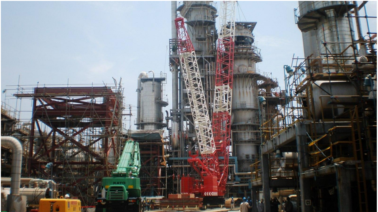
Provision of one (1) unit 600-Ton Demag CC2600 Crawler Crane at Limay, Bataan, Philippines for lifting one (1) unit Cyclone Assembly weighing 165 MT, with dimension of 7.6m(D) X 12m(H) and lifting height of 55m at Petron Refinery.
