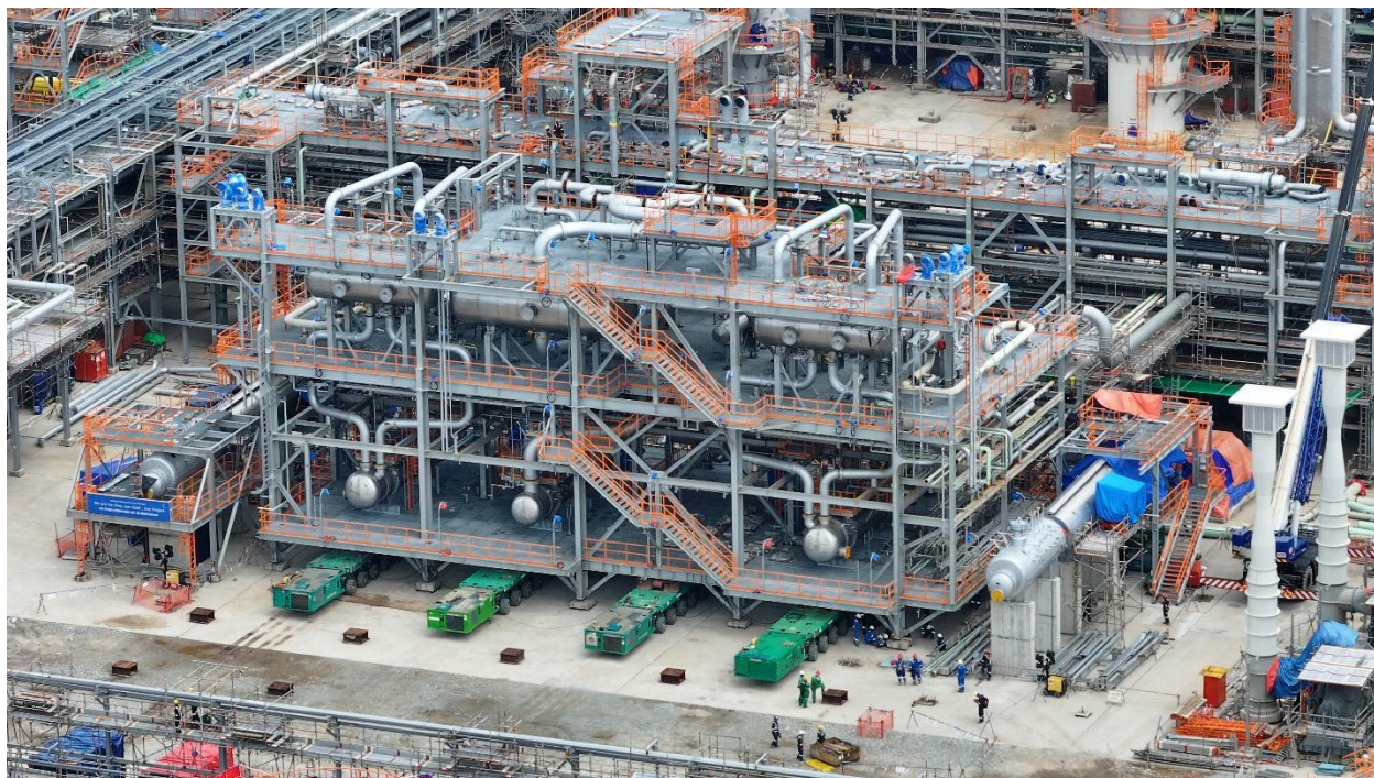
Load-in operation of 840 MT module from MOLF jetty at Bintulu utilizing 30 x 2 axleline and 2 PPU SPMT and transport to OGP site. Upon arrival, the configuration of the SPMT changed to 18 x 4 axleline and 4 PPU to manoeuvre into the highly congested area. The final installation is completed by jacking down onto permanent support ensuring perfect alignment and load transfer to the foundation.
