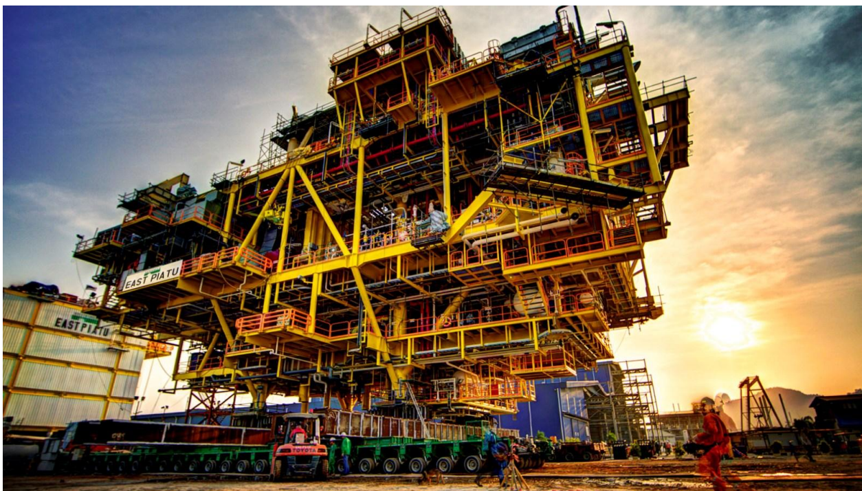
Shifting, Weighing, Load Out and Barge Ballasting for Newfield Peninsula Malaysia INC's CPP Topside with combined weight of 3500MT utilizing 120 axle-lines Goldhofer Self-Propelled Modular Transporter.
