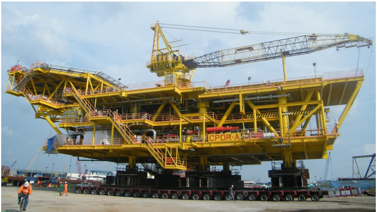
Shifting and loadout of CPDR-A Topside weighing 1958 MT for Cili Padi Gas Field Development Project at Kencana Yard, Lumut utilizing 72 axles Goldhofer PST-SLE and PST-ESE Electronic Multiway Steering System Modular Transporter on the 19th September 2010. Ten (10) units of ballast pump were used on the offshore barge to maintain stability during the cross-over.
