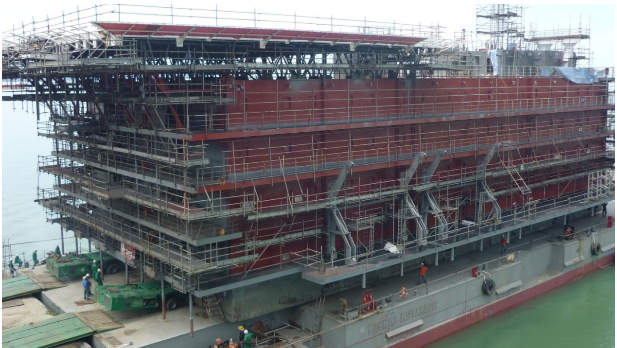
Shifting and Load out of a 2000 MT Accommodation Unit (H-131) onto a 111m Accommodation Barge in Boustead Penang Shipyard (BPS), Pulau Jelajak, Penang on 21 May 2011. A total of 2 x 36 - axle lines single file of Goldhofer THP combined with PST Self Propelled Hydraulic Controlled Modular Transporter.
